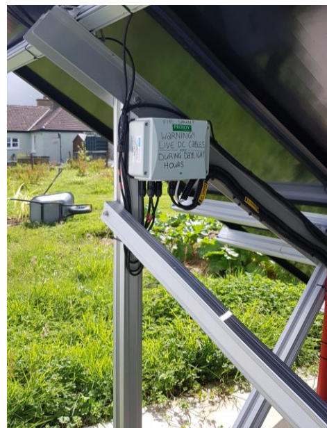
Automatic isolation located within 1.5m in cable length of the modules on a ground mounted installation.
