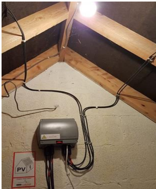
Automatic isolation located within 1.5m in cable length of entry to the building on a roof mounted installation.
