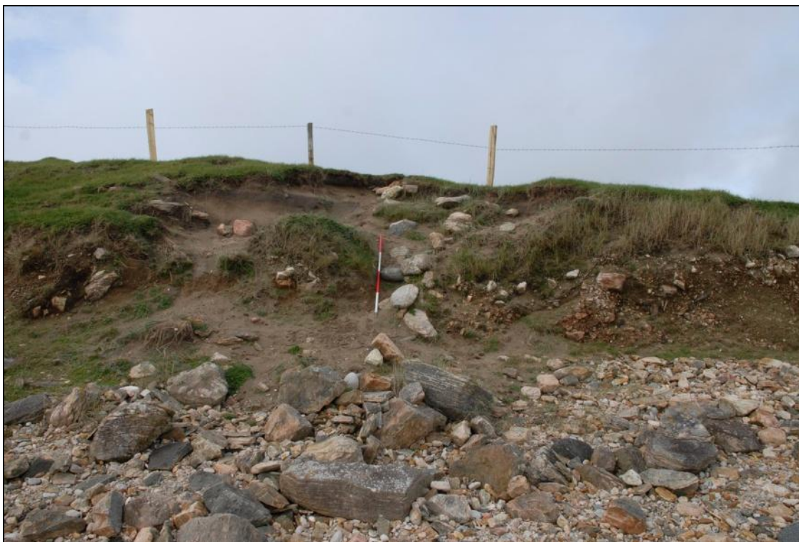
Plate 3. View of collapsing stone wall at RMP MA:016:07 Ballymacsheron Promontory
