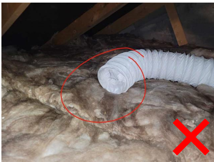
Figure 5: MEV Terminating within Attic Space
