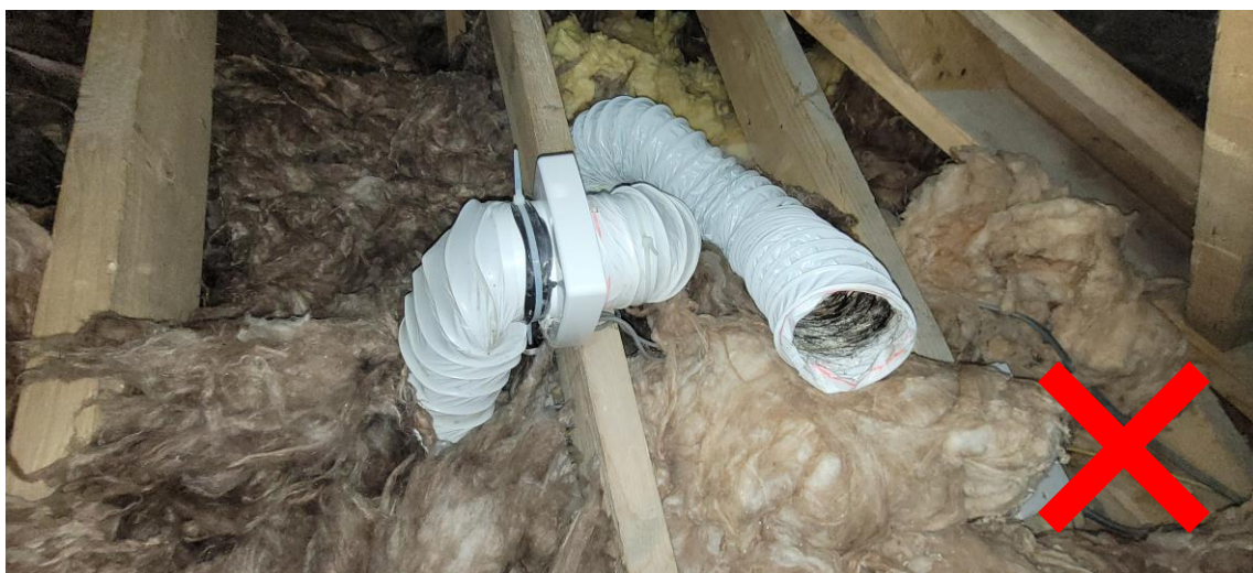
Figure 4: MEV Terminating within Attic Space
