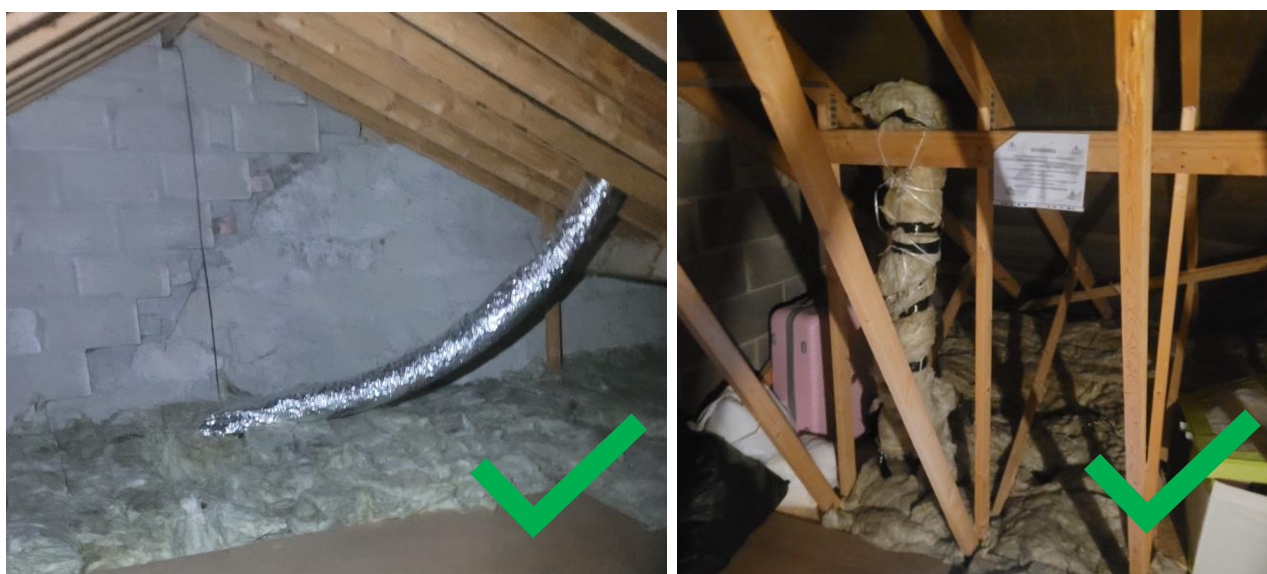
Figure 7: MEV ventilation ducting correctly to ventilation roof tile
