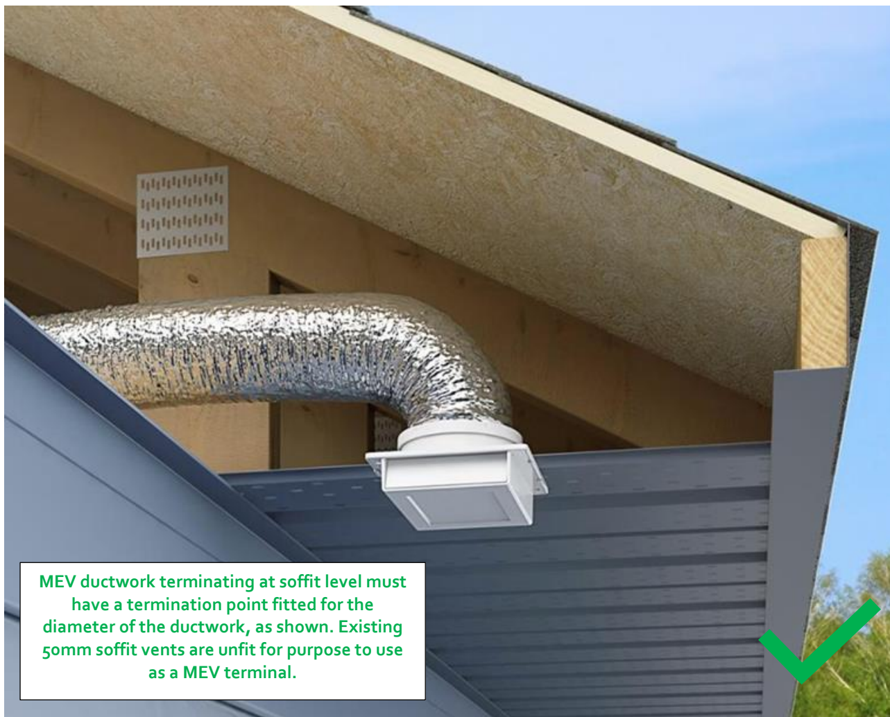
Figure 6: Compliant Roof Soffit Vents Installed for MEV Termination
