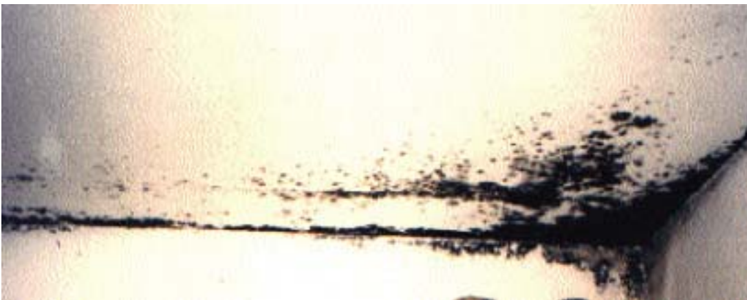
Figure 91 - Mould at external wall and ceiling junction
