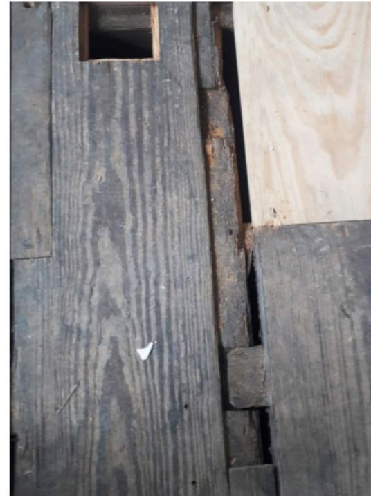
Figure 38: Care must be taken when lifting existing floorboards to conserve historic detailing like this biscuit joint
