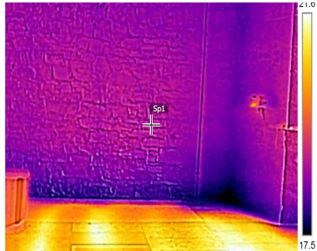
Figure 10: Thermal image showing additional heat flow at vertical and horizontal junctions with the abutting walls and floor. Note that the corner is the coldest point because it loses heat in three dimensions
