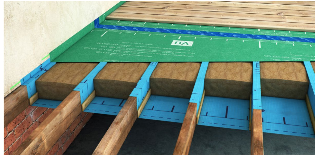
Figure 40: Slightly oversized batts of hemp insulation fit between joists over a wind-tight vapour-permeable membrane (blue) and beneath the intelligent vapour-control membrane (green). The vapour control membrane should be sealed to wall all round underneath the skirting. The sub-floor void should be cross-ventilated in accordance with TGD F and all pipework appropriately insulated
