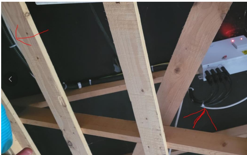
Fig 2: AC & DC cable tied together, not to COP. Simple separation is required
