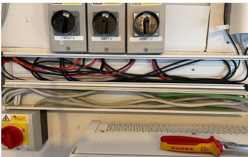
Fig 3: AC/DC run in separate trunking
