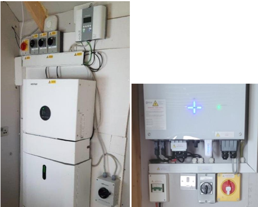
Fig 1: AC and DC cables not segregated
