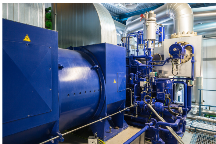
Figure 5.5: Steam turbine in a bioenergy plant
