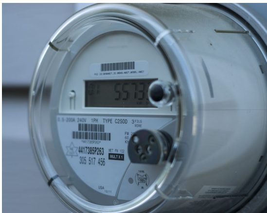
Figure 8.2: Electronic power meter
