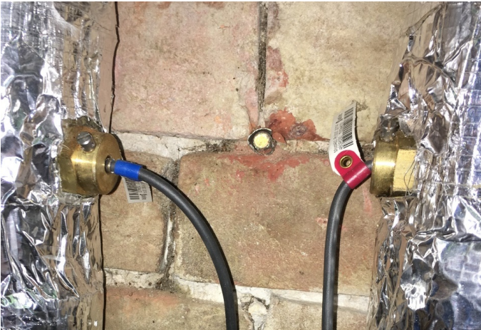
Figure 7.3: Matched pair of heat meter temperature sensors on flow (right) and return (left) pipes
