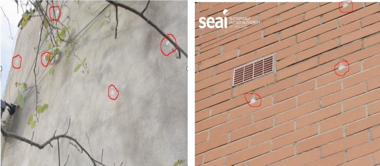
Figure 6 – Evidence of CWI
