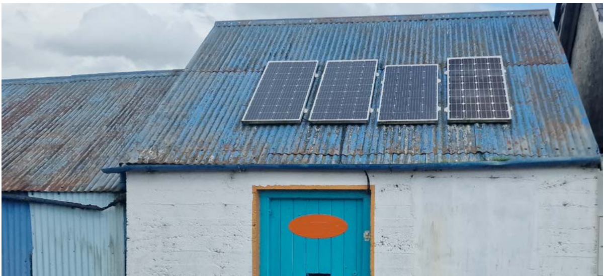
Figure 67: PV on the roof of an outbuilding
