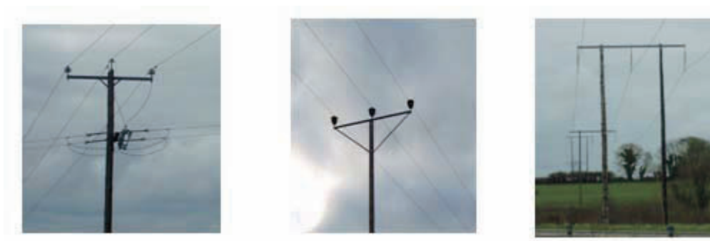
Figure 6-1: MV, 38 kV and 110 kV electricity lines using wood poles
