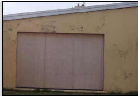
Plywood applied for security reasons
