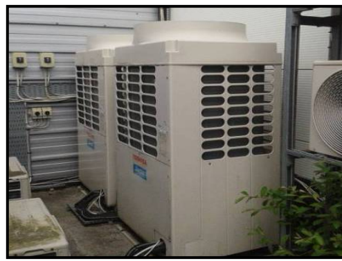
Multi-Split Outdoor units, (bigger than single split outdoor units)
