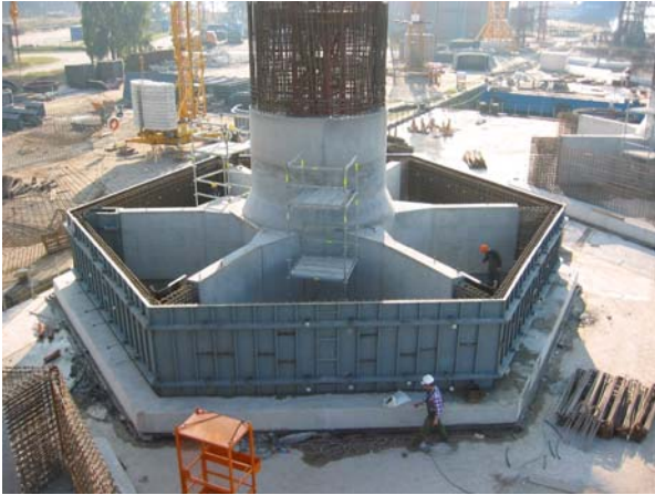
Figure 15: One of the gravitation foundations for Nysted offshore wind farm during fabrication on a barge. Ref [17]
