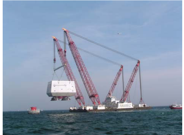
Figure 16: The 780 ton heavy transformer being lifted in place at the Nysted offshore wind farm. Ref [17].
