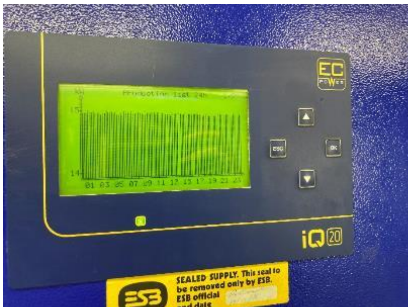
Figure 37: CHP power output over the last 24 hours
