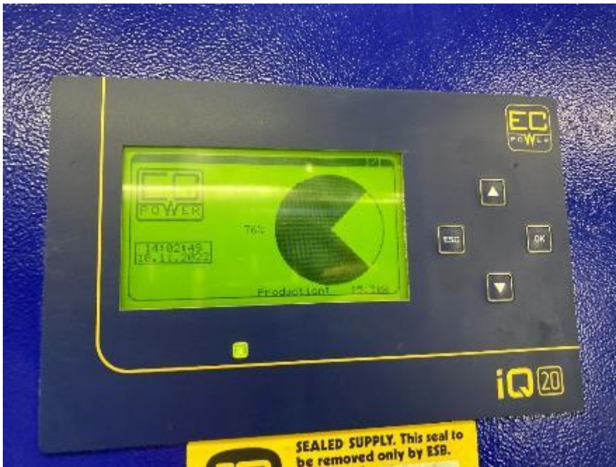
Figure 9: CHP electrical generation output screen
