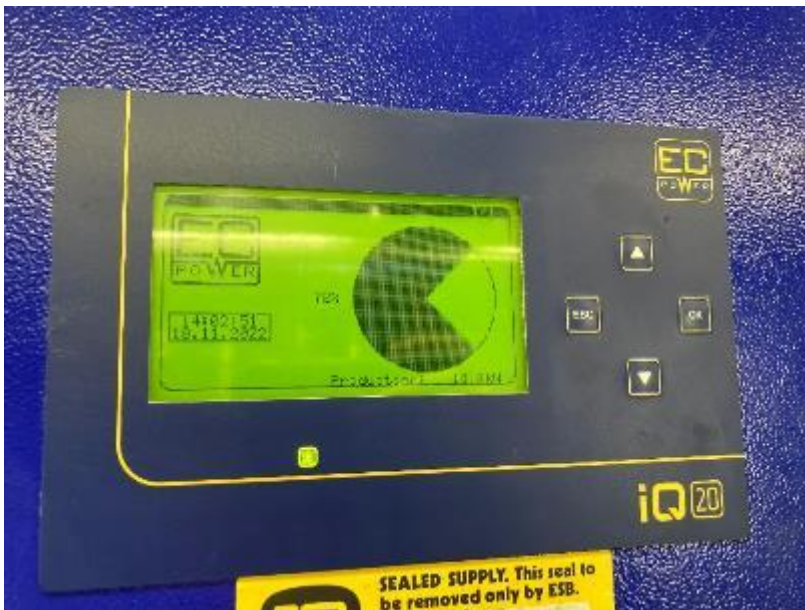
Figure 35: CHP electrical generation
