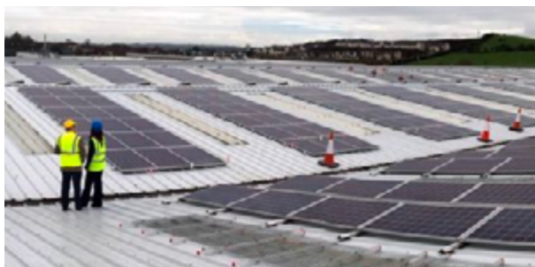
Figure 10: 300 kW installation at Kingspan Insulation
