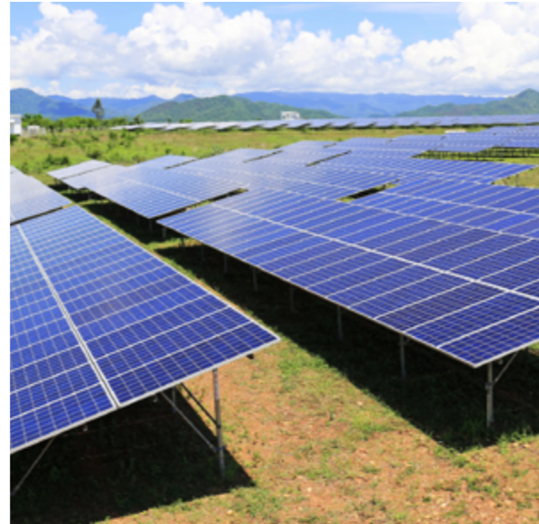
Figure 16: Ground-mounted PV on an Irish farm
