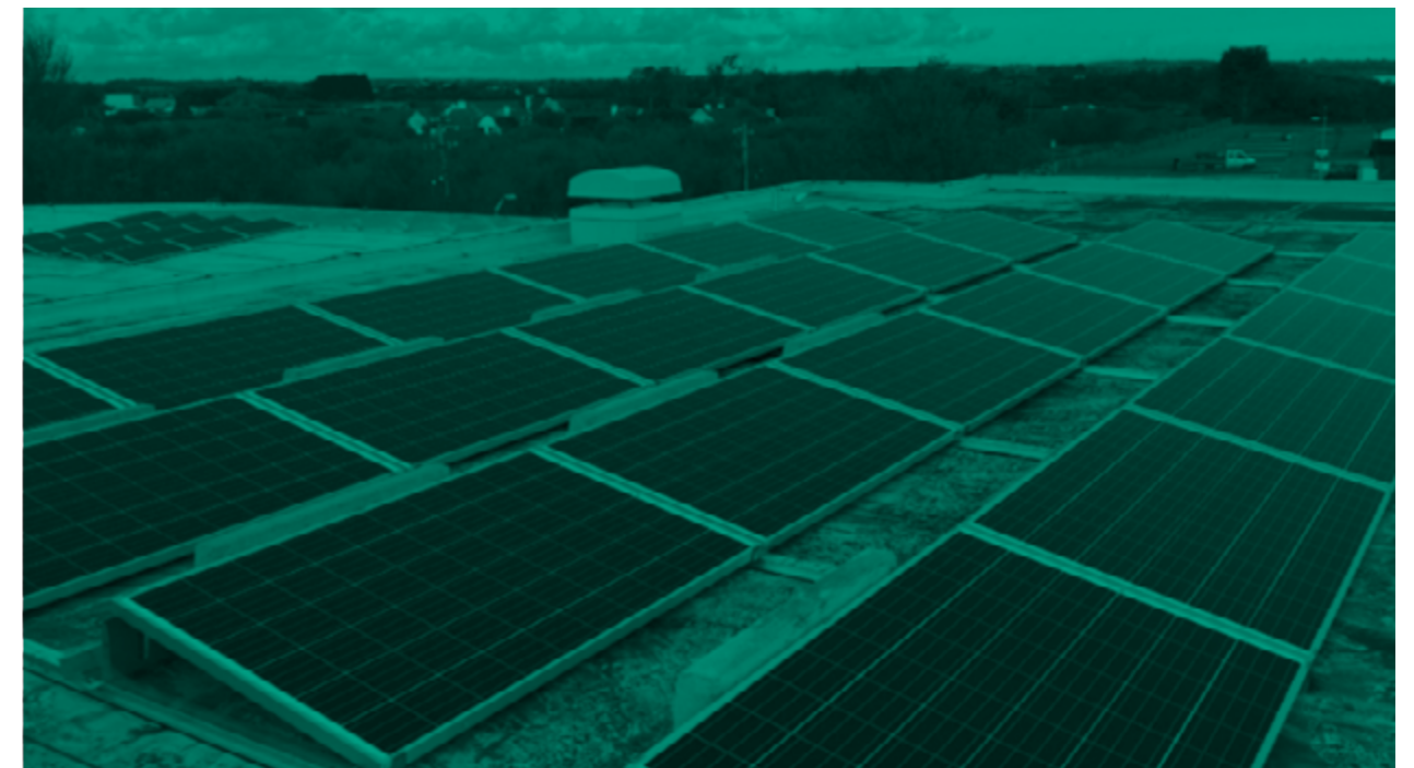
Figure 11: Rooftop solar PV on a leisure centre building
