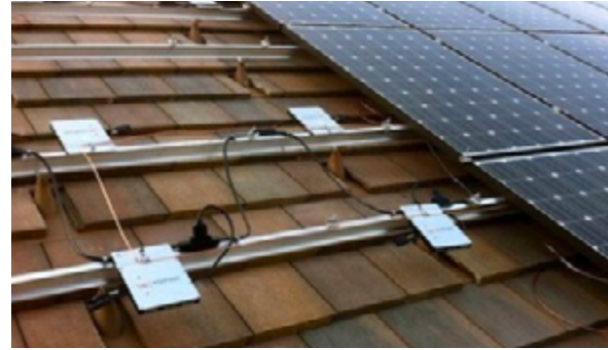
Figure 7: Micro-inverters installed under each individual PV module
